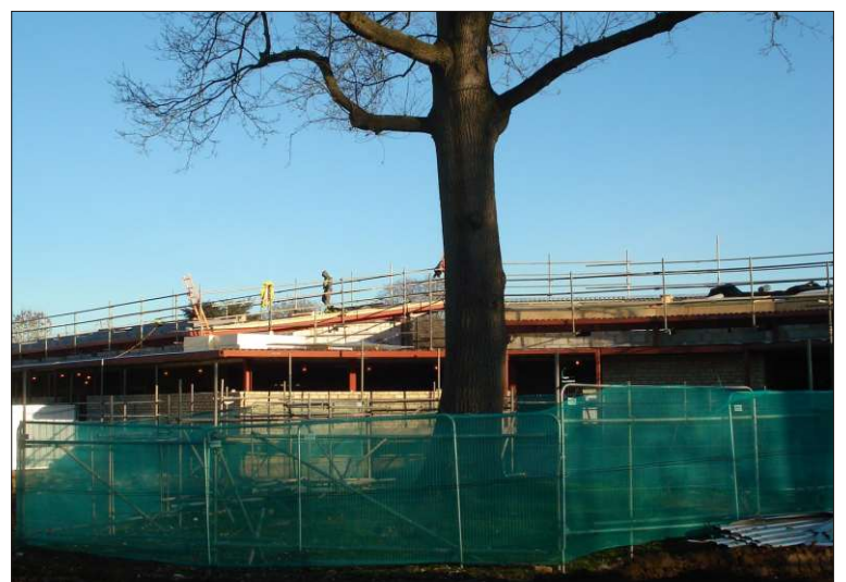
Construction of the new school around an old oak tree. Protective fences erected around the tree. October 2010.
